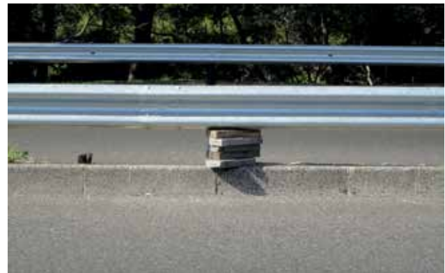
Barrier on wooden blocks
